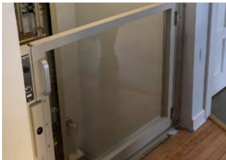
The newly installed interior lift at medical care respite facility at Sojourner House
